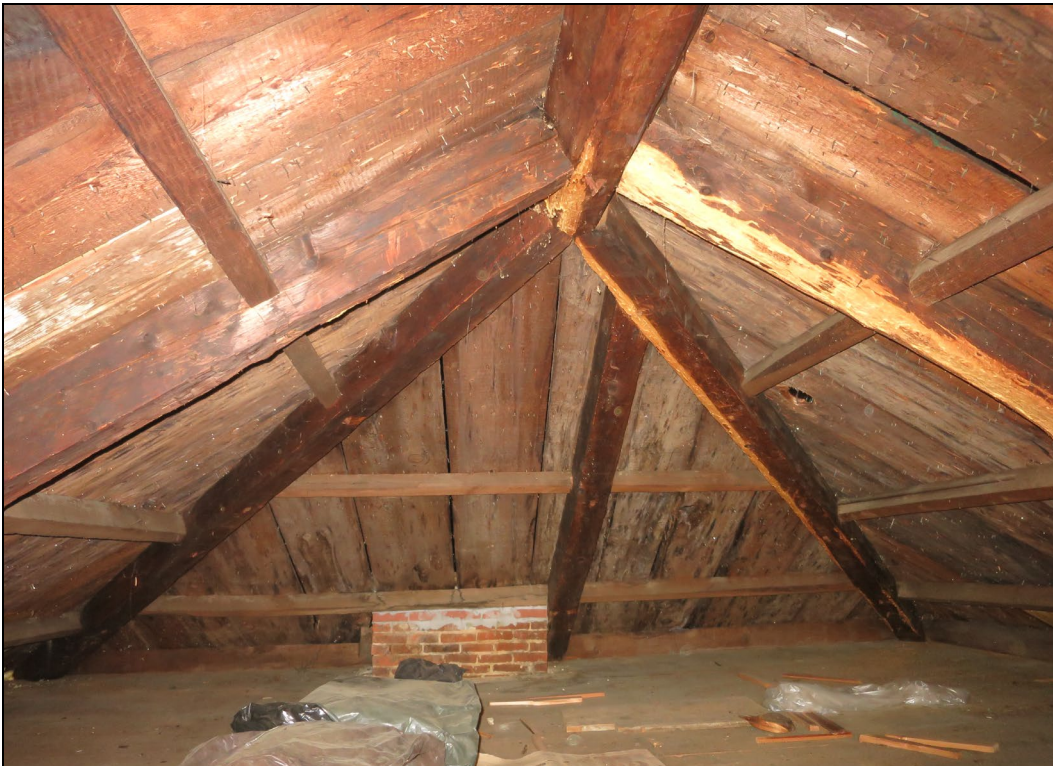
Attic, looking east showing ridge beam, principal rafters & common purlins at hip junction.
