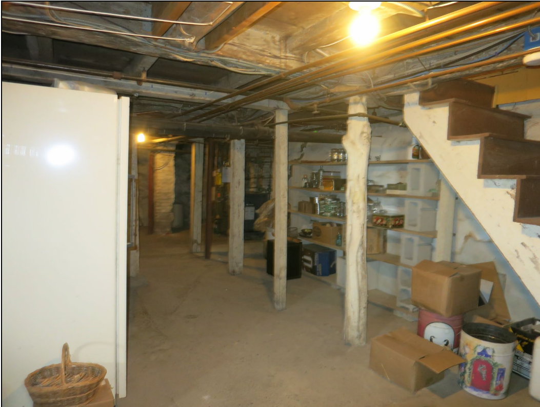
Basement looking west in front section showing posts supporting wall where saltbox joins.
